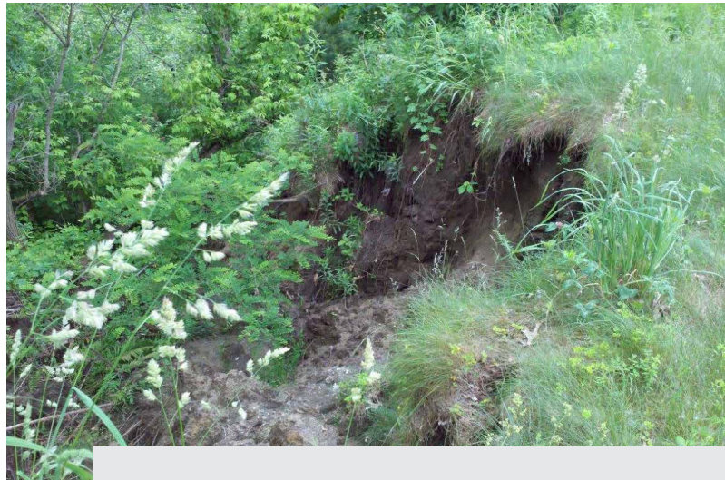
Erosion from Improperly Draining BMP
