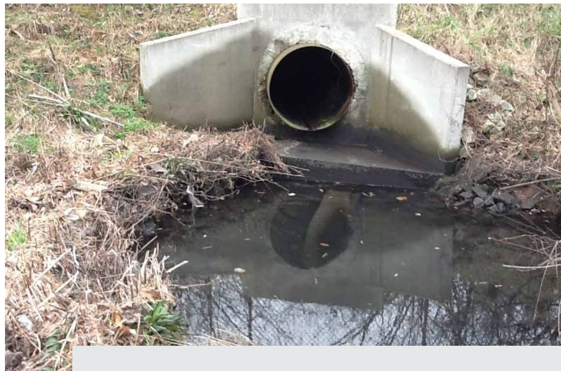
Erosion at Outlet
