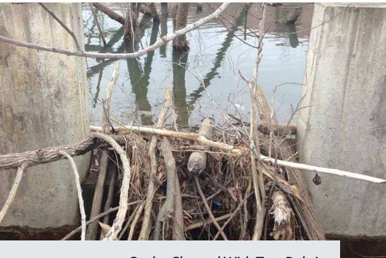
Outlet Clogged With Tree Debris from Beaver Activity
