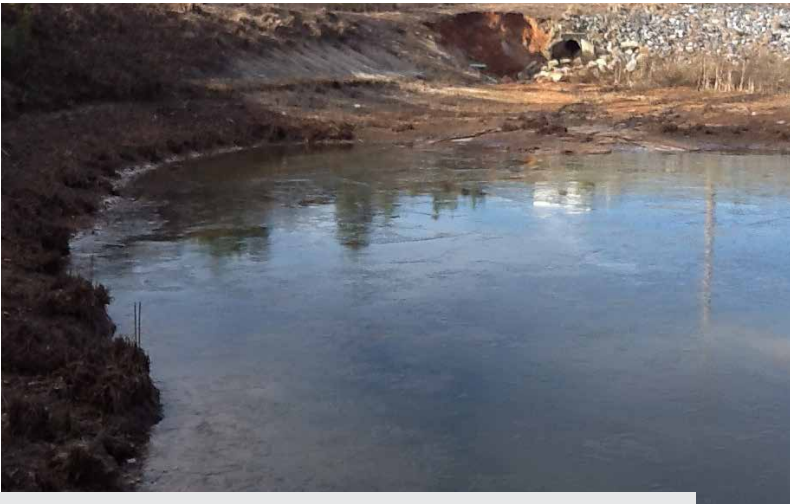
Severe Erosion at Inlet
