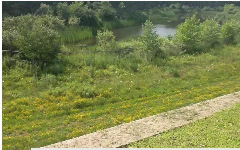
Overgrowth of Vegetation at Retention Pond
