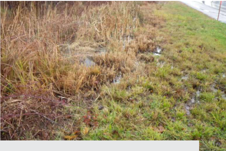
Swale with Excessive Vegetation
