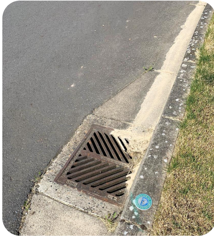
Illicit Discharge of Paint to the City's Stormwater System in 2022
