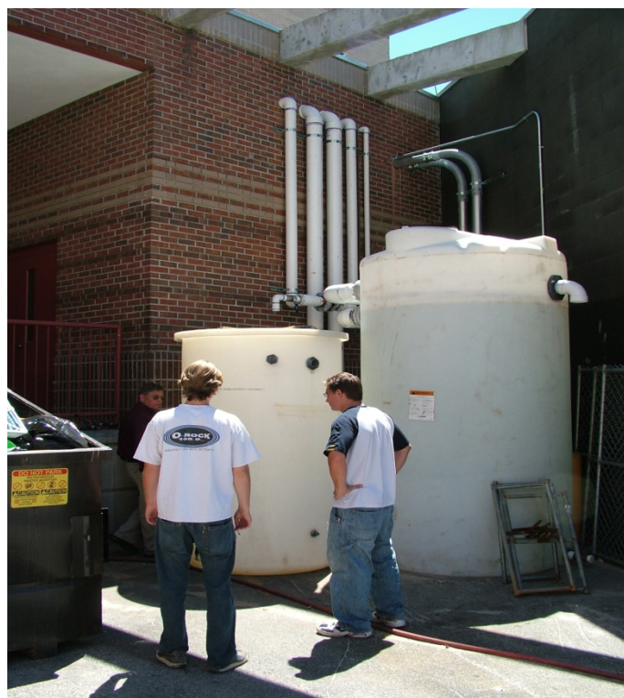
Figure 3.4-2 Example of Above-Ground Industrial Cistern Storage
