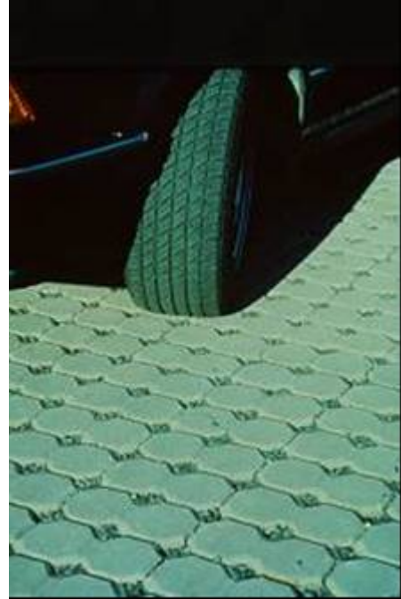
FIGURE 4-17 Parking Lot with Interlocking Concrete Grid Installation (Courtesy of the Interlocking Concrete Pavement Institute)
