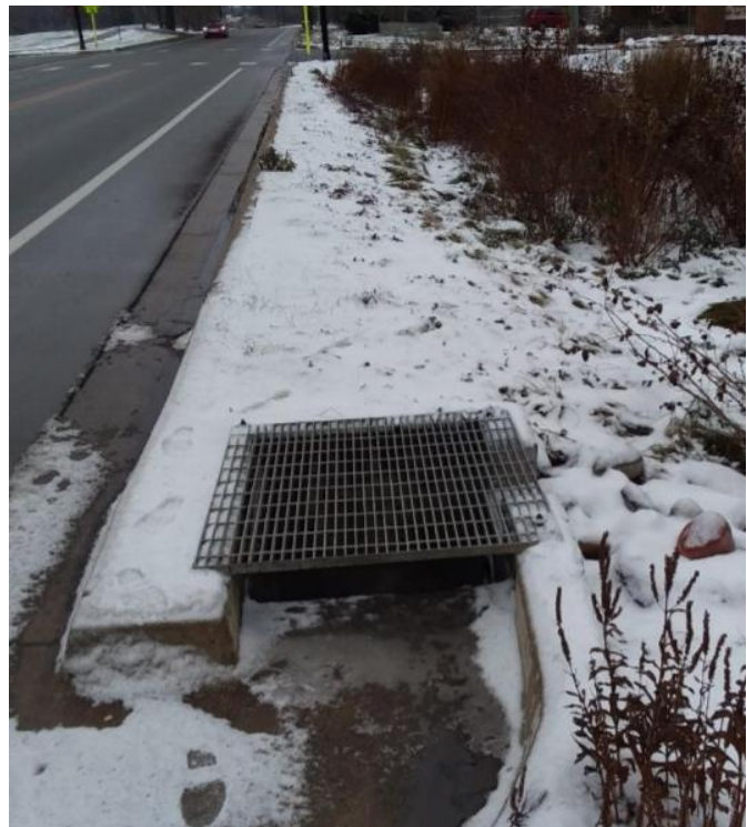
Figure 8-10: Inlet Sump Structure (source: City of Ann Arbor)
