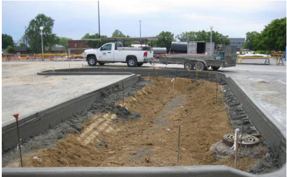
Figure 8-12: Construction of Bioretention Cell in Parking Lot, Evansville, IN (source: Indiana Office of Community & Rural Affairs)
